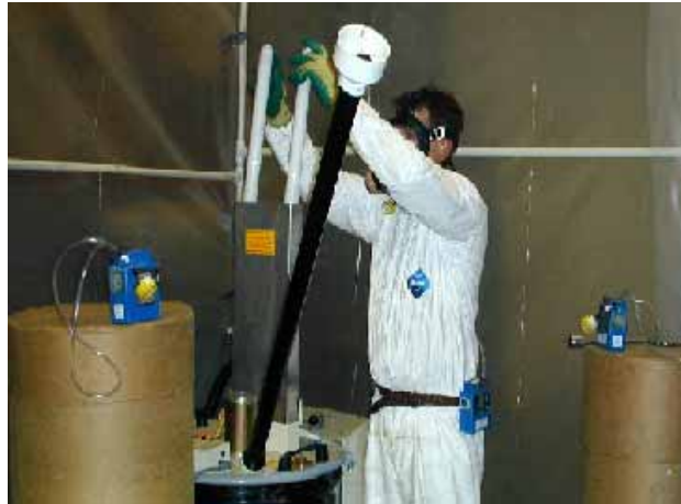
Photograph 3. 6: Crushing of U-Tubes - Manufacturer C Device
